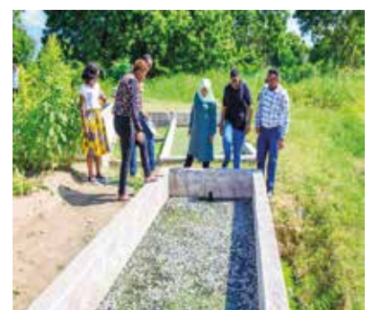
Wastewater Treatment Plant at UDSM
